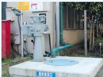
Valve for cutting off rain sewage in case of abnormality
