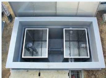
Oil-water separation tanks adopting the double-structure system
